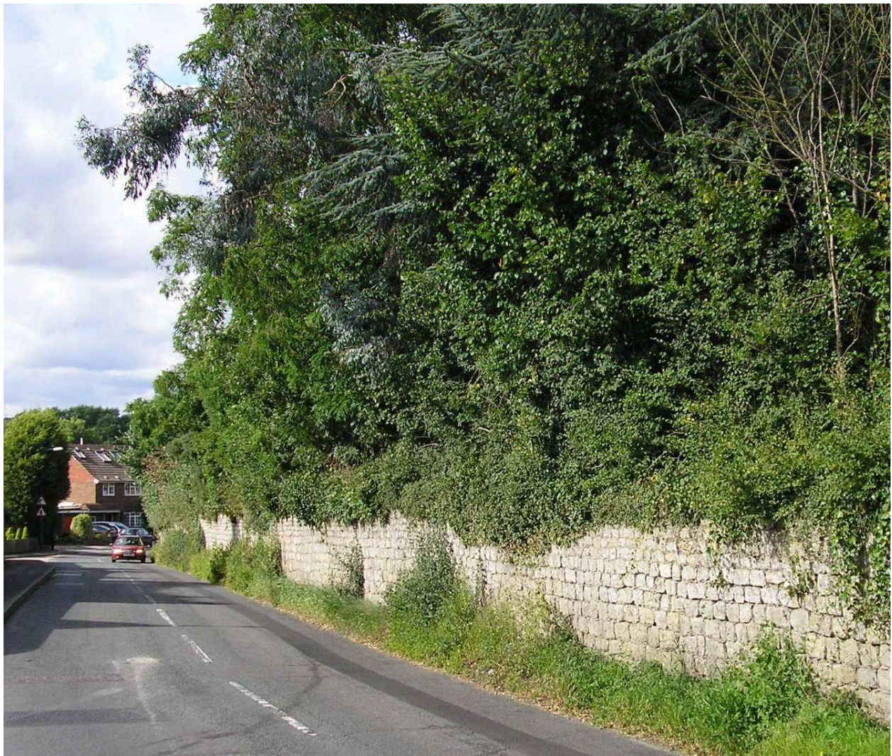
An important feature of Homedean Road is the planting and this long coursed ragstone wall.
